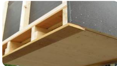
There is a difference in thickness between the plywood and the hardwood bottom board.
