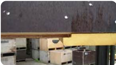
The bottom of the pallet on the box is closed with 9 mm plywood.
